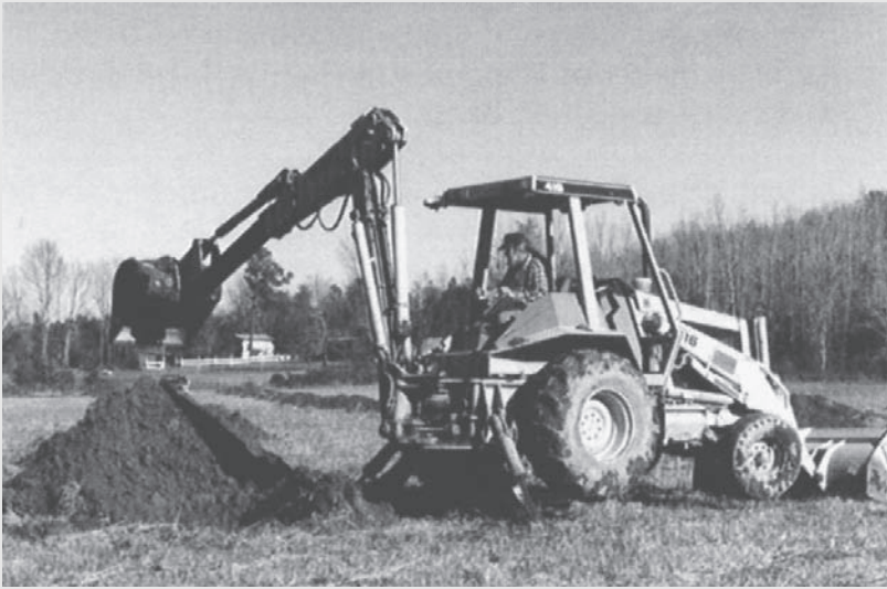
Figure 5.3. Small backhoes often are used to dig deeper test units, strip areas, and even help backfill. Rental usually is by the day or half-day, depending upon the area, with the cost including both the equipment and the operator. The kind pictured here is most common; the bucket arm will reach fourteen feet (a little over four meters). Bucket width usually is sixty centimeters. (Photo courtesy of R. Jerald Ledbetter and Southeastern Archeological Services, Inc.)
